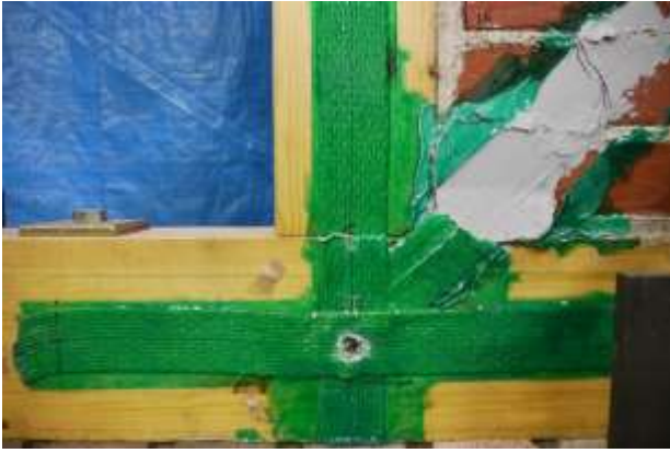
Figure 12: Fracture of the AFRP sheet on the front side of the bottom connection (TFM-CH-AFRP)
