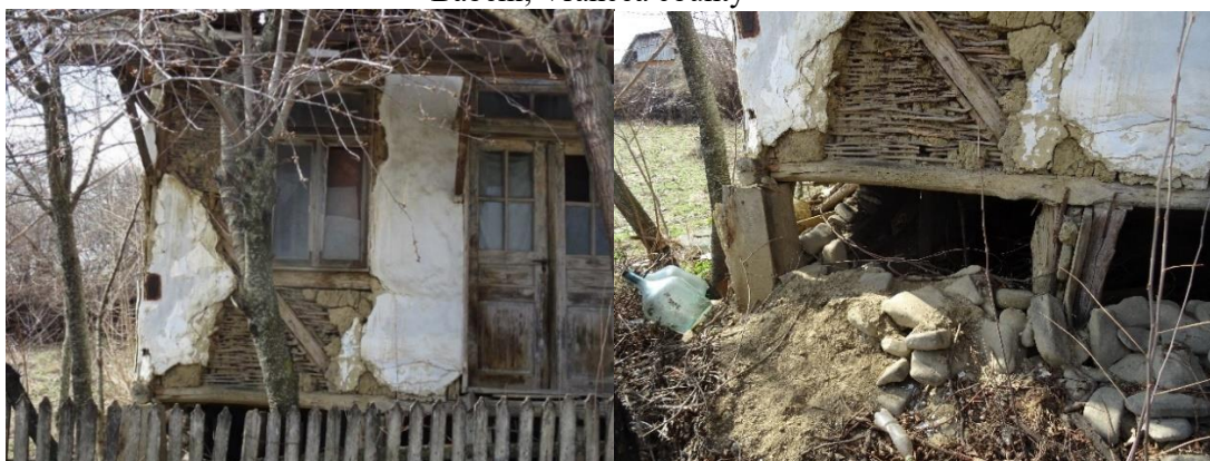
Figure 12: Details of traditional house with timber skeleton and wattle and daub (Type 3) over 100 years, from Băbeni, Vrancea county
