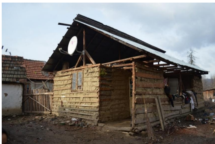
Figure 13: Building with timber and earth with straw infill structure (Type 4), from Viperești, Buzău county
