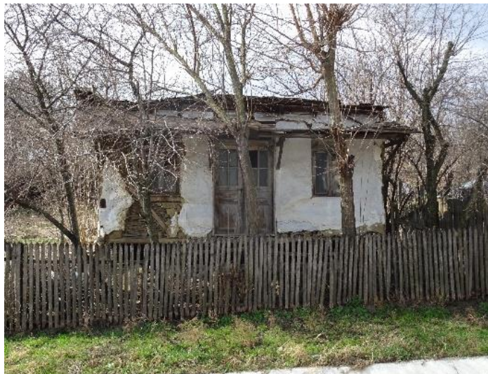
Figure 11: Traditional house with timber skeleton and wattle and daub (Type 3 – ”grădele”) from Băbeni, Vrancea county
