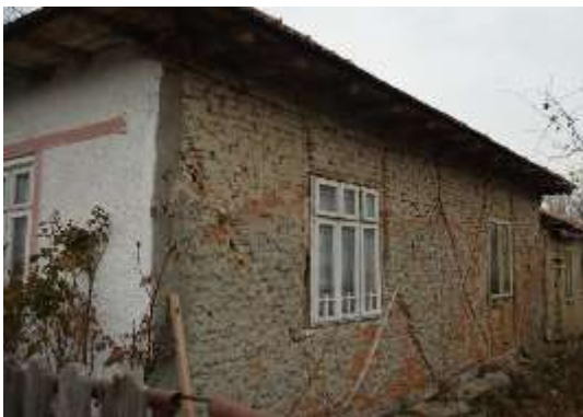
Figure 7: Building with timber and brick masonry infill structure, from Viperesti commune, Romania, built in around 1925 with unreinforced masonry, and reconstructed after November 10 th , 1940 major earthquake with timber frames and infills – backyard façade
