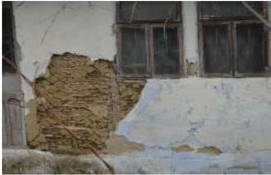
Figure 11: Building with timber and wattle and daub infill structure, from Viperesti commune, Romania, built in around 1910-1920 – detail infill
