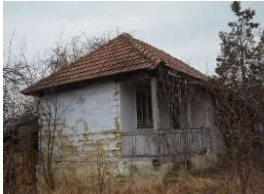
Figure 8: Building with timber and earth with straw infill structure, from Viperesti commune, Romania, built in around 1930-1940 – main façade
