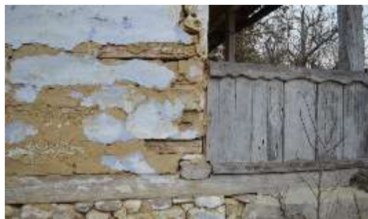
Figure 9: Building with timber and earth with straw infill structure, from Viperesti commune, Romania, built in around 1930-1940 –infill detail
