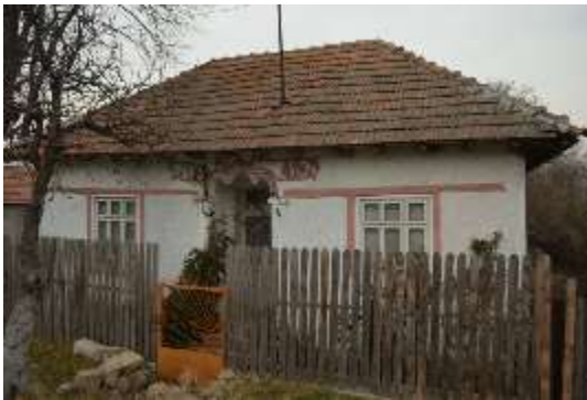
Figure 6: Building with timber and brick masonry infill structure, built in around 1925 with unreinforced masonry, and reconstructed after November 10 th , 1940 major earthquake with timber frames and infills – main façade
