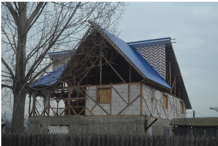
Figure 19: Building with timber skeleton and AAC (autoclaved aerated concrete) masonry infill (Type 5), from Viperesti, Buzau county
