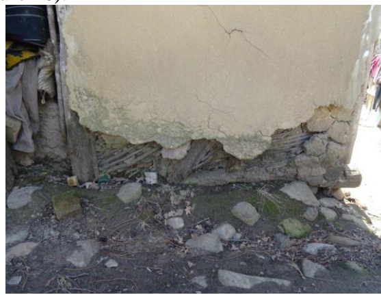
Figure 16: The bottom timber beam is simply sitting on the ground
