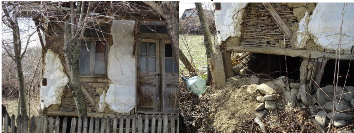
Figure 12: Details of traditional house with timber skeleton and wattle and daub (Type 3) over 100 years, from Băbeni, Vrancea county
